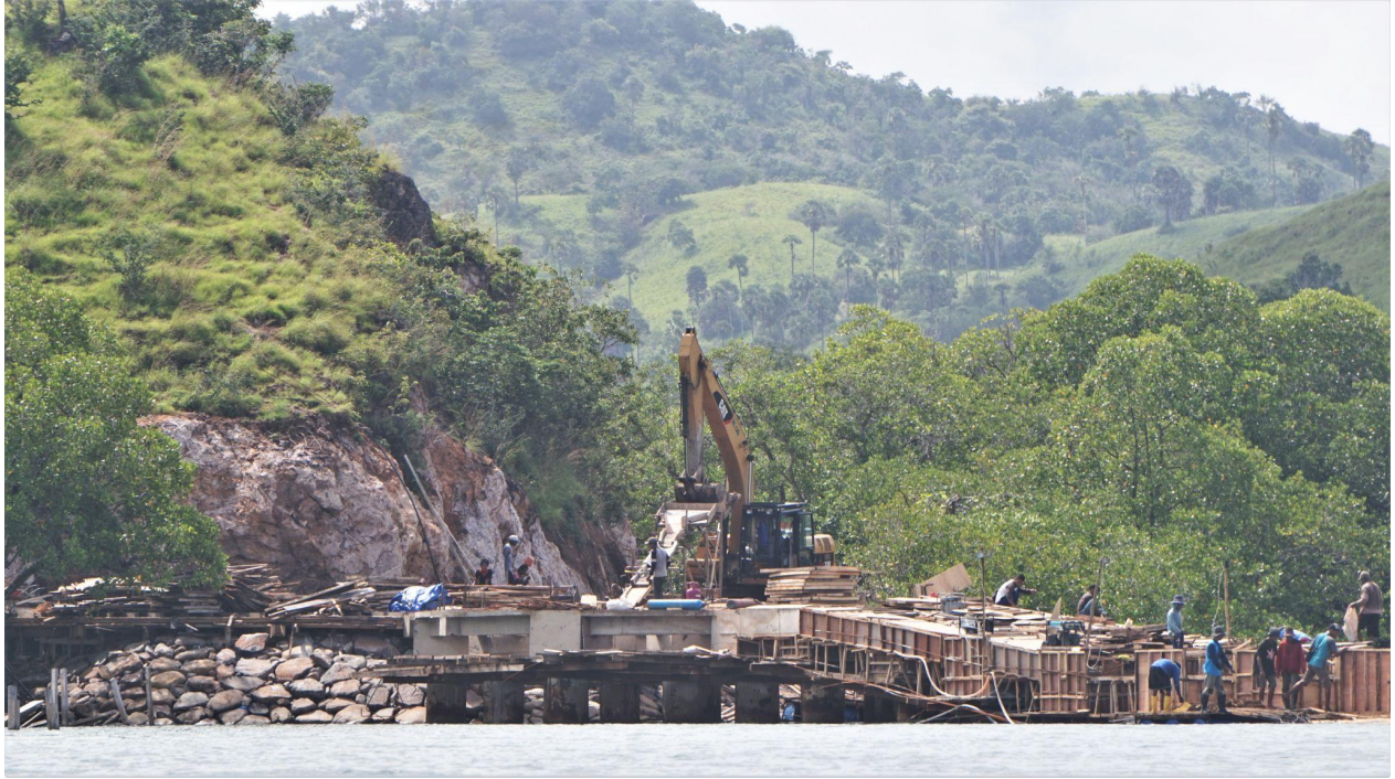
Fig. 5: Construction process still continuing on Loh Buaya, Rinca island. Photo: WALHI NTT, 2021
